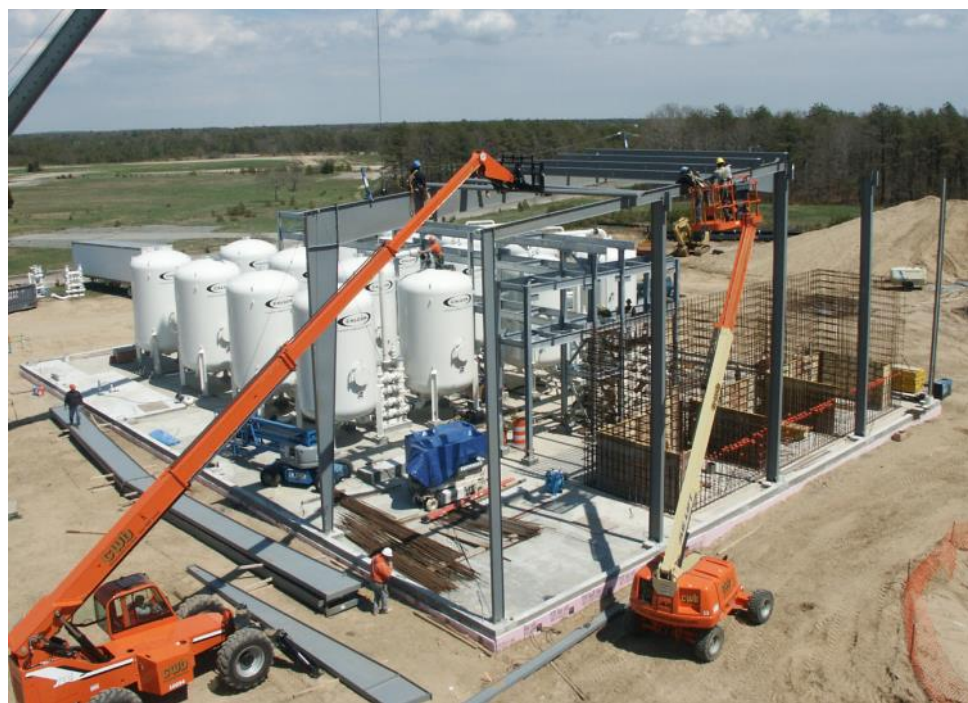
Construction of the Air Force’s largest groundwater treatment facility on JBCC with 16 vessels each containing 20,000 pounds of GAC. The cleanup system treats contaminated groundwater that comes from several plumes on and off-base including CS-21 via extraction wells and pipelines. Cleaned water is then returned to the groundwater aquifer.
